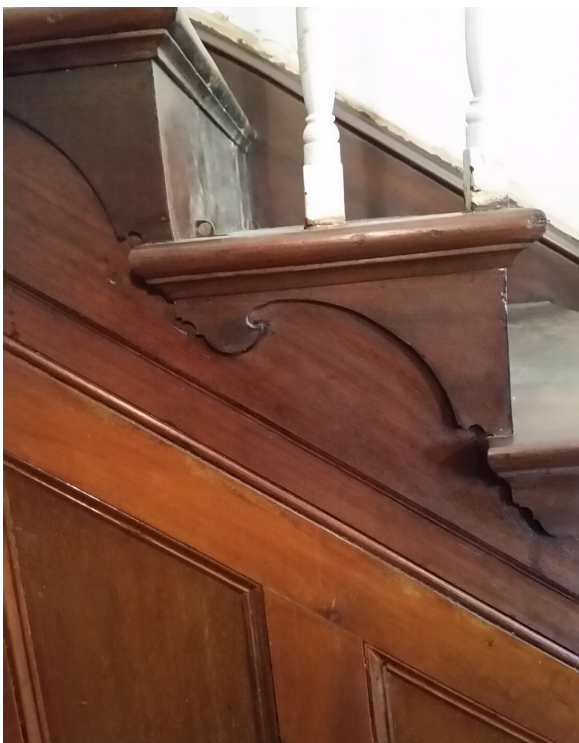
The new stain on the treads, contrasting with the orange hue of the Estapol coat on the side panel.
